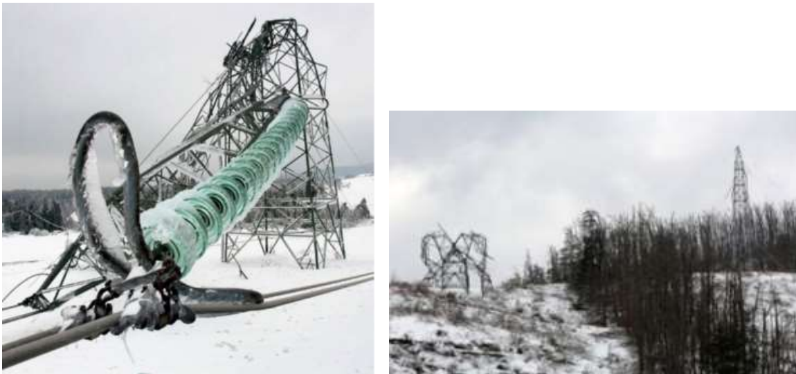
Fig. 2 Typical image of a 400 kV OHL tower after catastrophic icing storm (TSO, ELES) [3].
