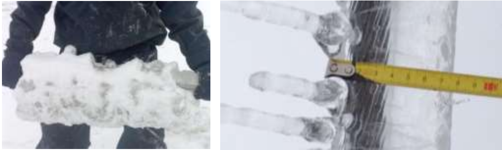
Fig. 1 Glaze ice on a conductor on the OHL 110 kV Cerkno – Idrija (TSO, ELES) [3].
